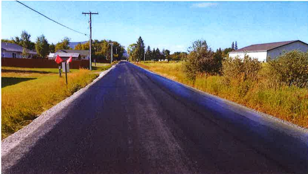
Substantial Completion – A new roadway surface on the North end of Main Street.
