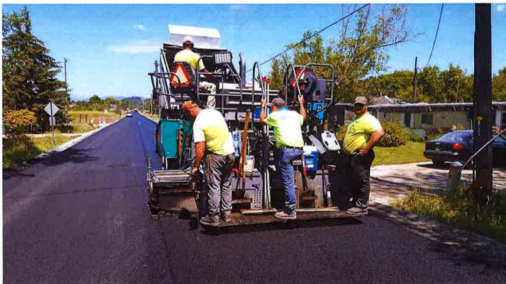
Wood's Crushing and Hauling placing the final lift of asphalt on Main Street.
