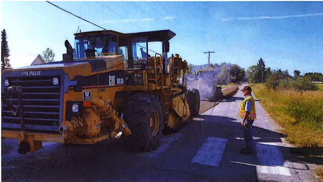
Highway District and Bonner County crews working together to build a road within the City.
